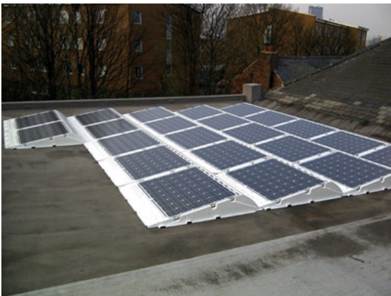
Figure 3: Roof Mounted Photovoltaics
